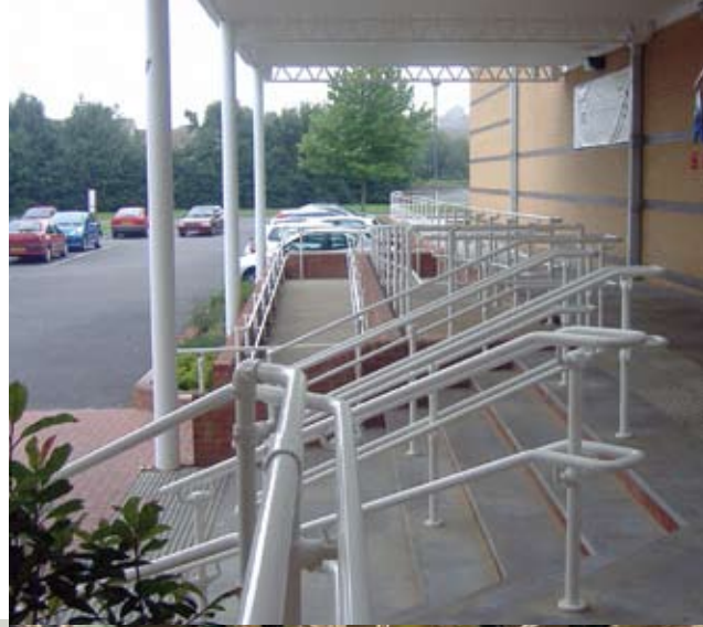
Right: ADA Compliant Railing for Public Access
